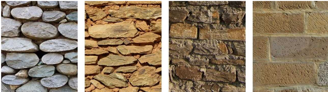
Fig. 3 - Different stone masonries: a) round river boulders with mud mortar; b) random rubble stone masonry with mud mortar; c) random rubble stone masonry brought to courses with cement mortar; d) ashlar stone masonry with lime-sand mortar (courtesy of SSF).
